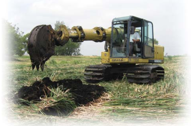
Mr. Jim Hering of Thornton Equipment Services, Inc. Using Gradall 2200 with Nyrim® Track Pads Removing Drain Tile.
